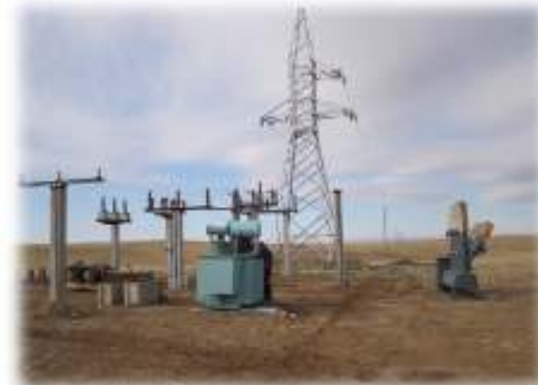
35KV / 1,250 KVA substation on site
