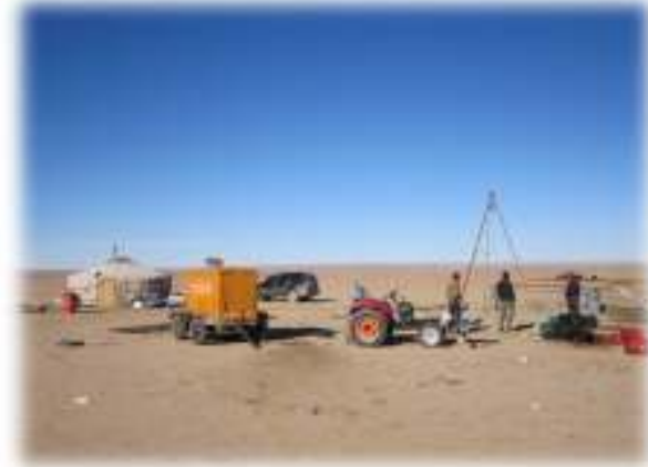
Bore hole at industrial-use water reservoir
